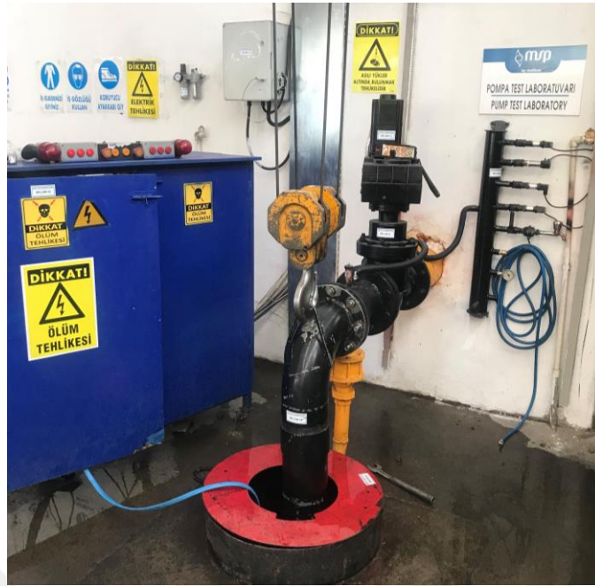
Figure 6.16 Servo-controlled valve, pressure sensor, flowmeter, and auxiliary tank arrangement
