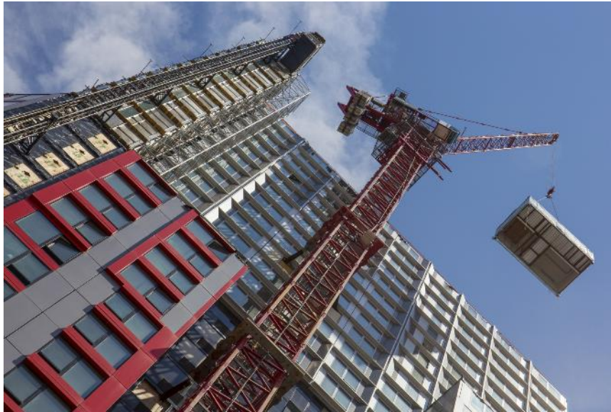
Figure 4.2.23 B2 Tower during construction, lifting a module by crane (B2 | SHoP, n.d.)
