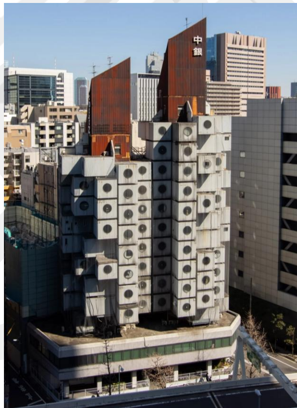
Figure 4.4.6 Demolition process of the Nakagin Capsule Tower ( Demolition of Iconic Nakagin Capsule Tower Begins in Tokyo , n.d.)
