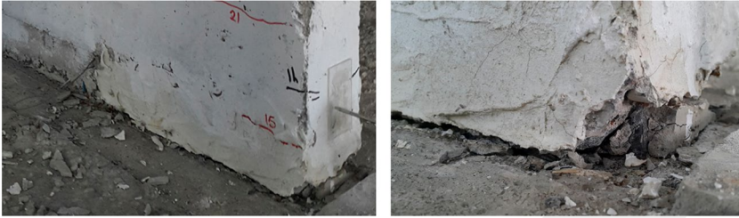
Fig. 11 Buckling of the reinforcement of the shear walls and separation at the base of the shear wall in the strengthening of the intact frame test
