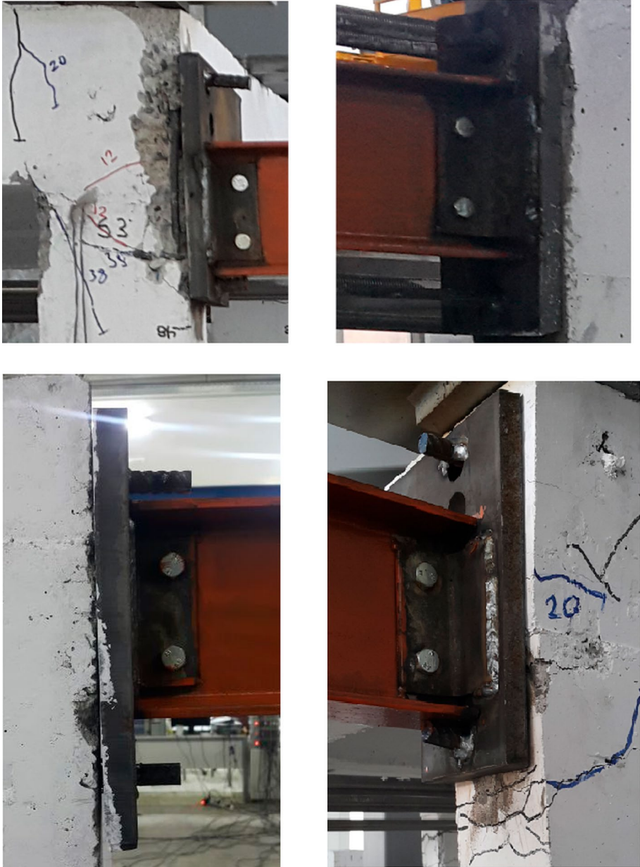
Fig. 12 The anchors for the steel tie beams in the damaged frame strengthening test
